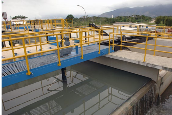
STP Porto Novo in Caraguatatuba (North Coastal Region) is one of 36 certified with ISO 140001
